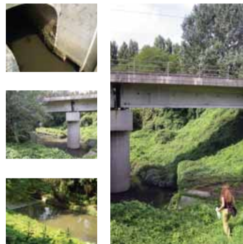
outlet of the polluted Fossetta River into Roncajette park; the water is contaminated with wastewater and stormwater
